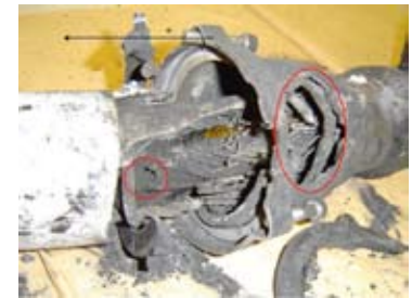
Undetected PD in a Cable Termination Results in Flashover
